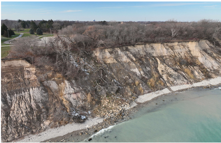
Warnimont Park Bluff and Coastal Erosion
