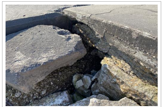
Damaged Concrete Cap and Revetment
