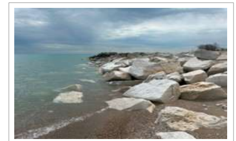
Stone Slope Displacements
