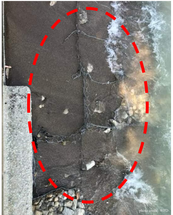
Damaged gabion baskets
