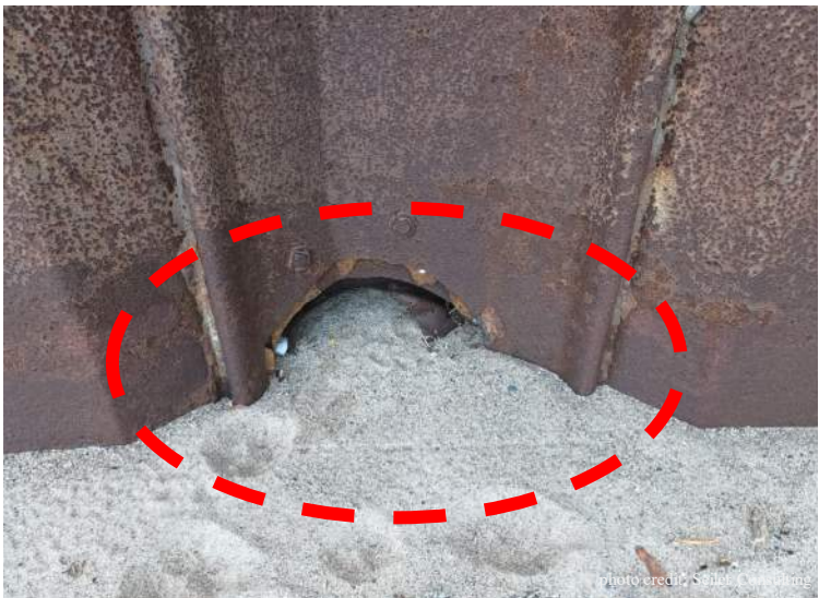
Damaged sea wall
