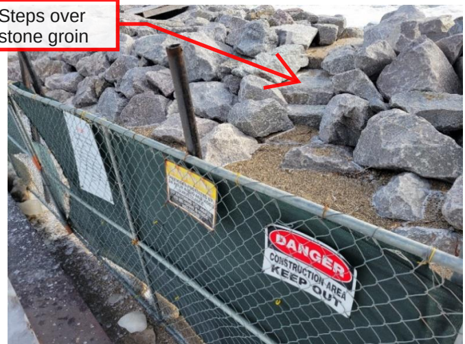
Steps over stone groin at 205 Sheridan, Feb-9-2025
