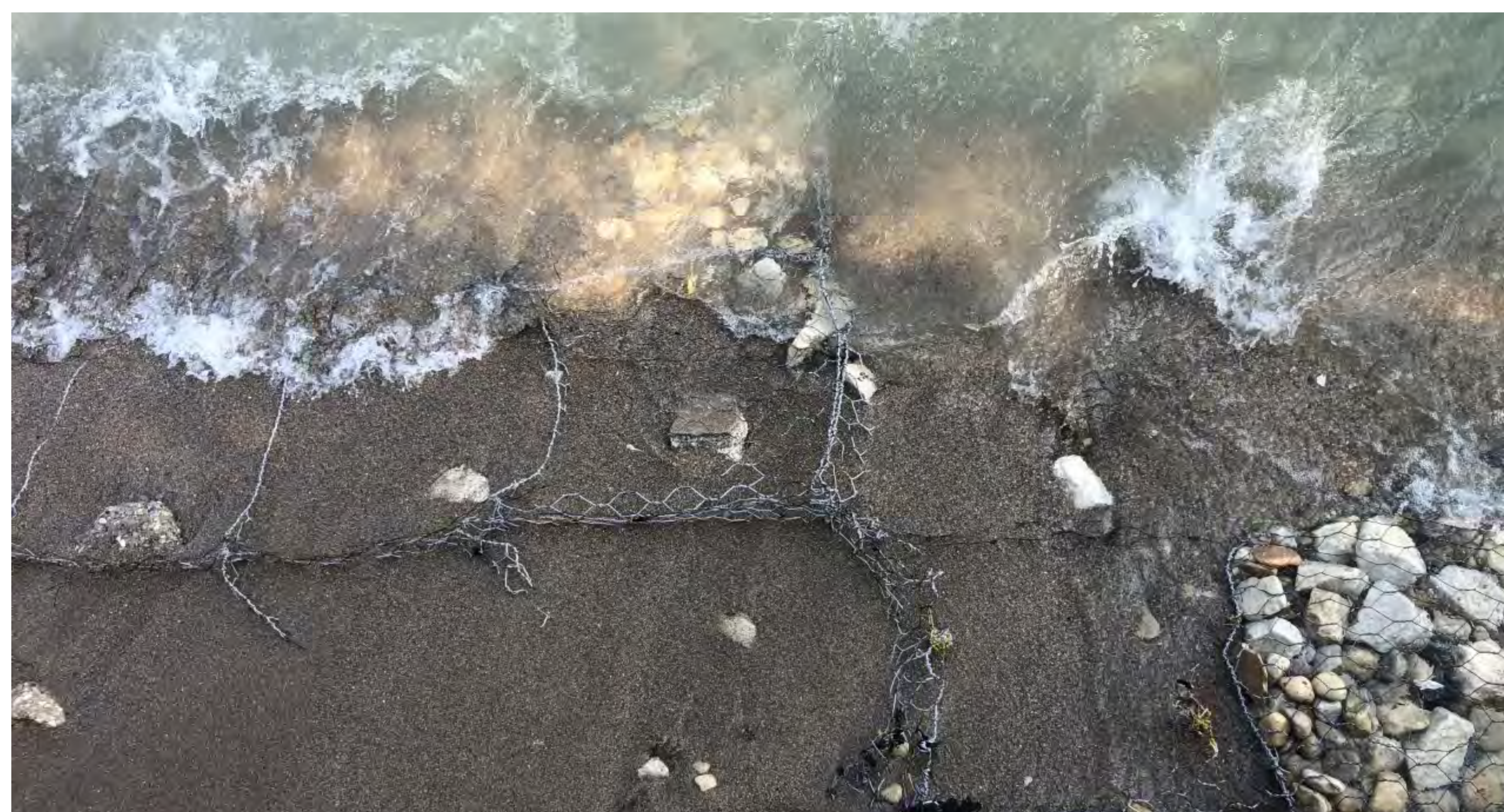
ELDER LANE | FAILING GABION BLANKETS OCTOBER 2020
