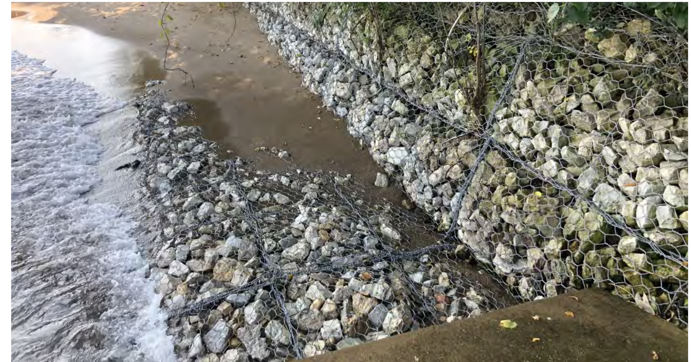
ELDER LANE | FAILING GABION BLANKETS OCTOBER 2020
