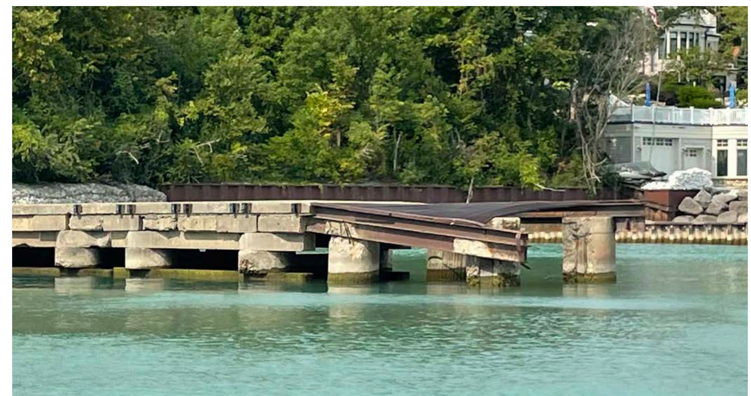
ELDER LANE | FAILING PIER SEPTEMBER 2020
