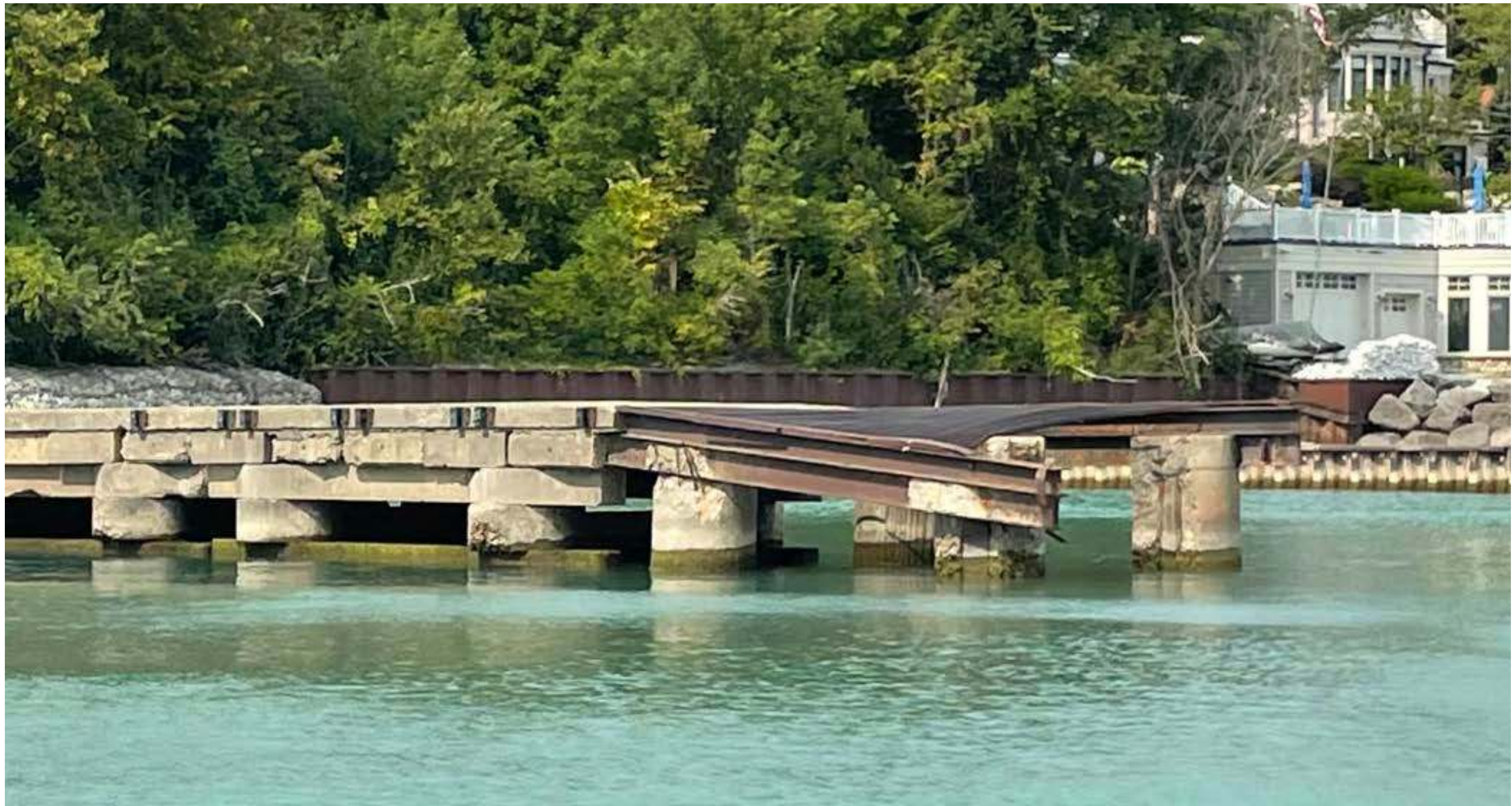
ELDER LANE | FAILING PIER SEPTEMBER 2020
