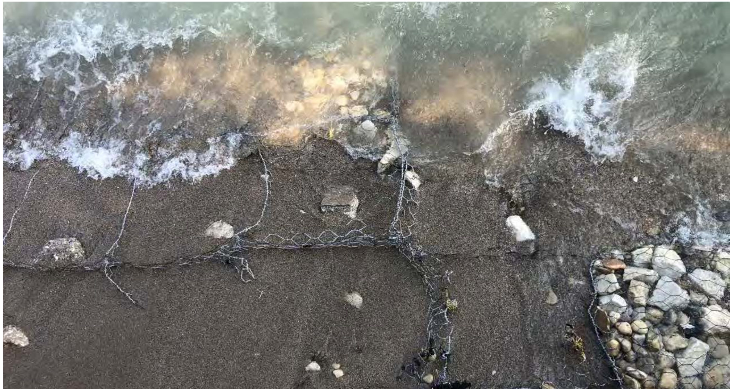
ELDER LANE | FAILING GABION BLANKETS OCTOBER 2020
