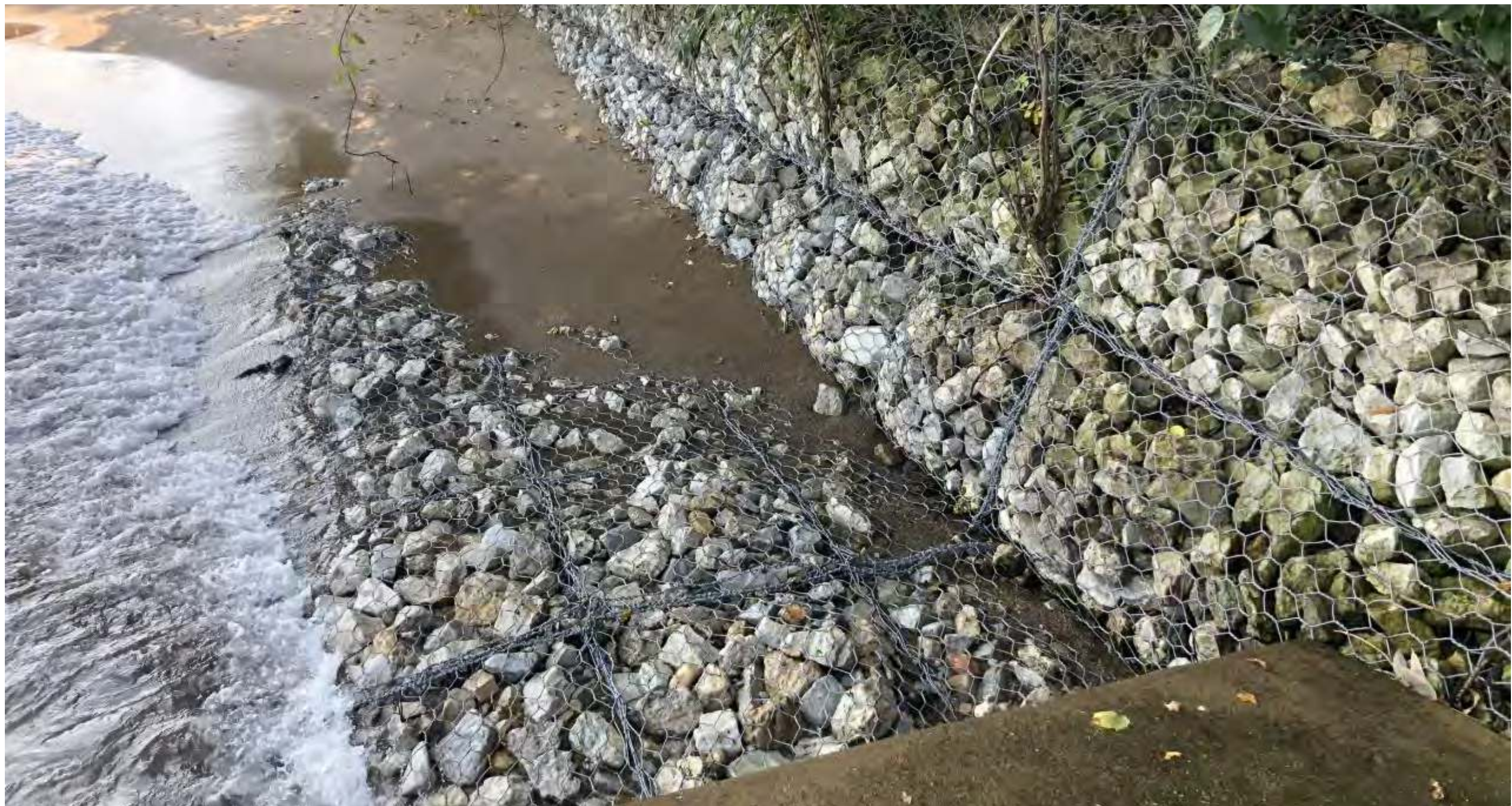
ELDER LANE | FAILING GABION BLANKETS OCTOBER 2020
